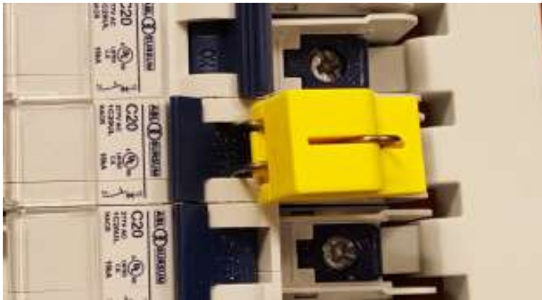
FIG 2 STEP 4 – LOCKOUT IN PLACE
