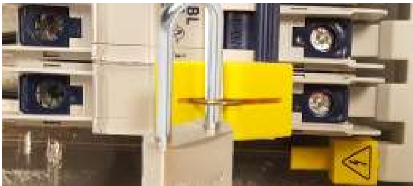
FIG 2 STEP 5 – BREAKER LOCKED OUT
